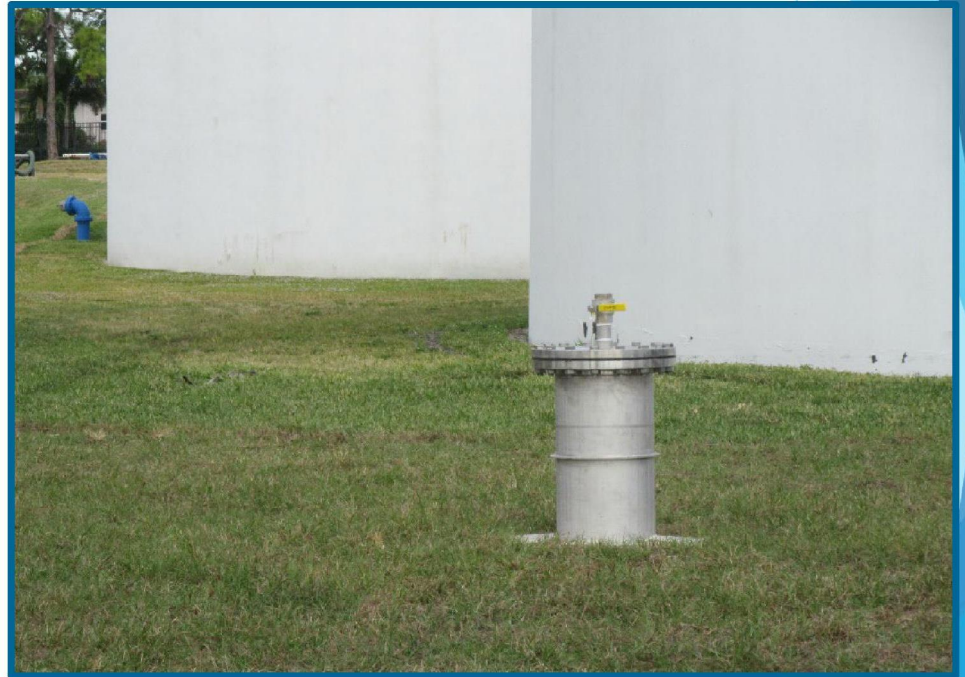
Floridan Aquifer Well FA-1
