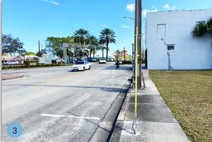
Figure 16 Images of sidewalk conditions within the study area.
