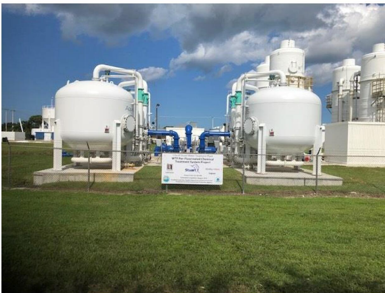
City of Stuart PFC Pre-Treatment Facility
