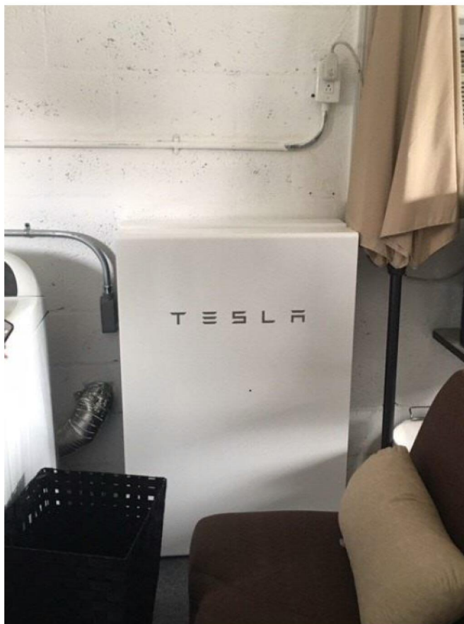
Residential Tesla solar power system
